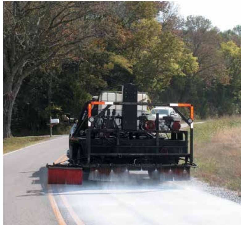
Contractor Pavement Restorations, Inc. places bio-based Delta Mist at an application rate of 0.10 gal./yd 2
