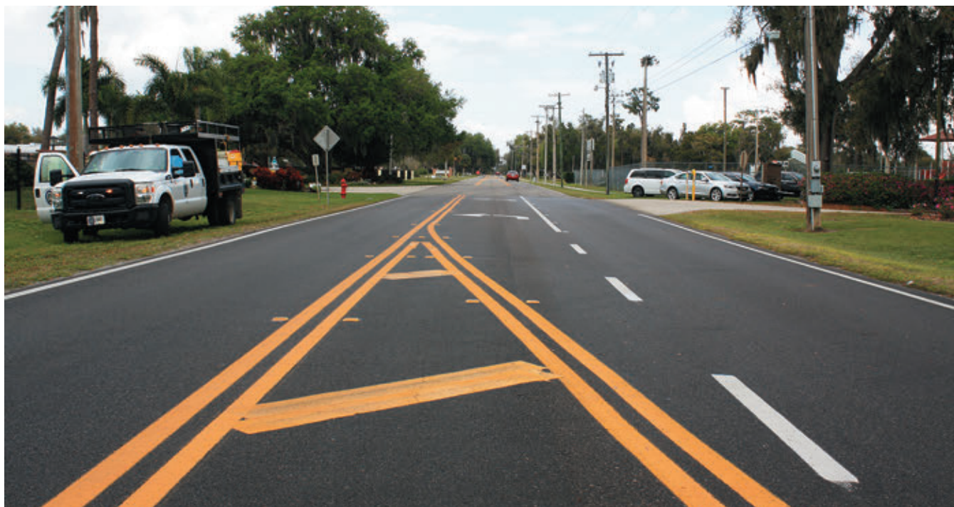
Delta Mist rejuvenator cures transparent and traffic can be returned after two hours
