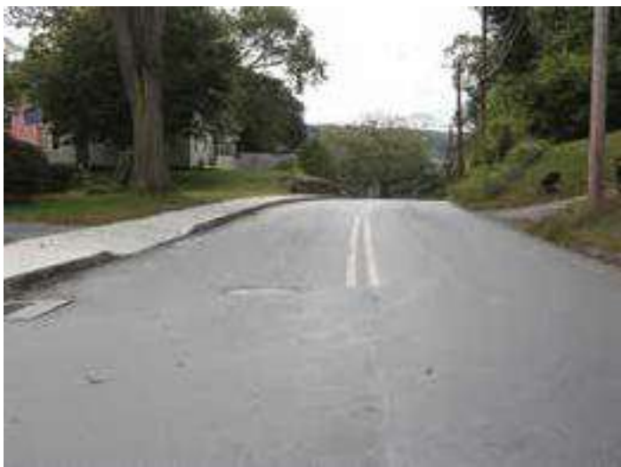
The rejuvenator went down white and cured clear in 90 minutes, allowing a return-to-traffic in that time. No restriping was required.
