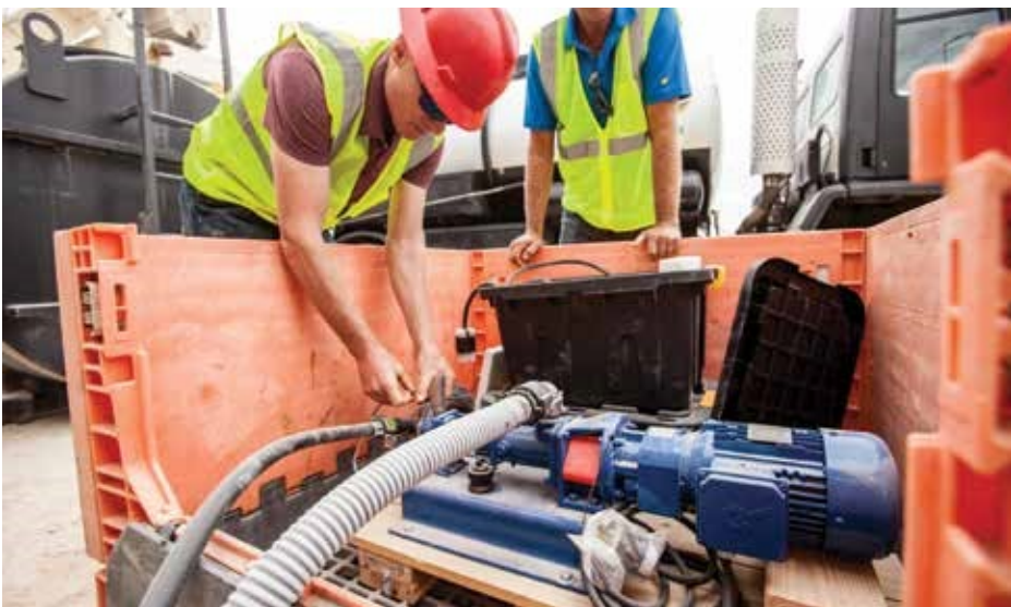
The Delta S is delivered in 275-gallon totes weighing about 2,200 pounds. Here the team working at CSA Materials set up the Moyno Assembly to pump Delta S into the plant at a rate of 1.64 gallons per minute. Steven Twining, a system technician for Rub-R-Road, Kent, Ohio, ran the pump to deliver the Delta S.
