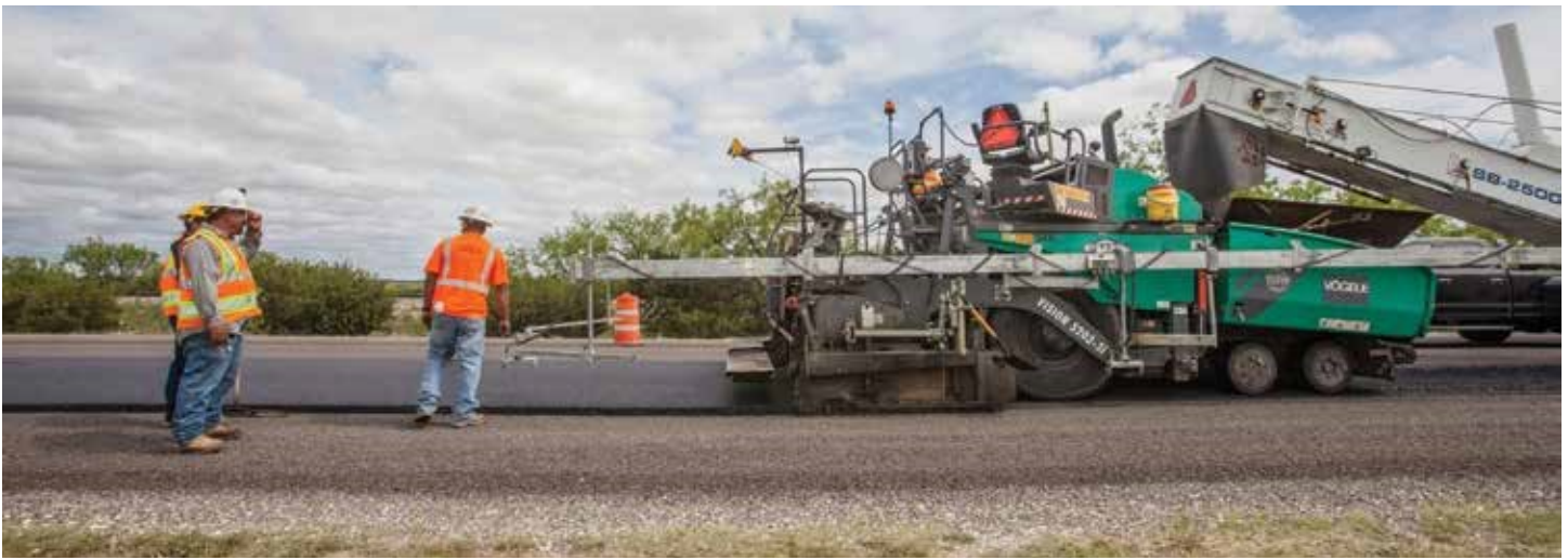
Each sub lot was approximately 400 tons, paved 2 inches compacted, produced at 275 degrees F.
