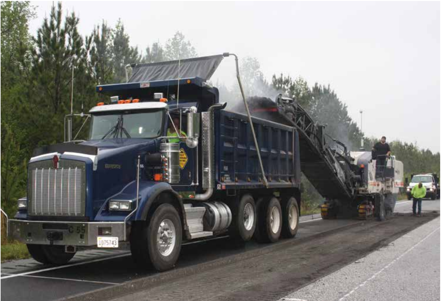
The failed wearing course of N7 was milled off to allow installation of the modified mix, which incorporated a PG67-22 binder, 35 percent RAP with Delta S rejuvenator, and no RAS. The modified mix was allowed extended storage time in the silo to eliminate the possibility of another failure due to reduced mix shear strength. This repair was completed the week of May 9, 2016, and ESAL testing resumed shortly thereafter.
